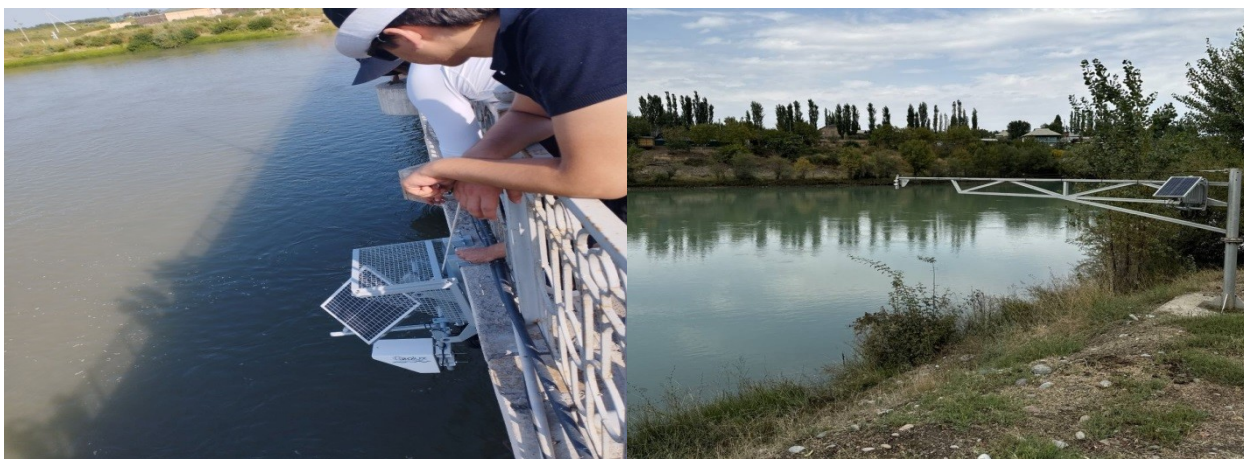
Figure 2. Automated water metering devices installed in Namangan region
